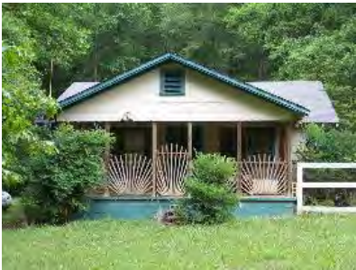
Porch with inappropriate addition of balustrade in an incompatible style.
