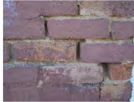
Crumbling Mortar should be repointed.
