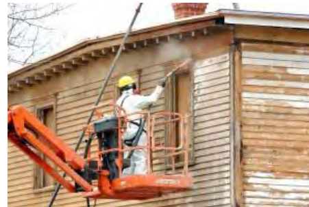
Cleaning wooden features and surfaces with destructive methods such as power washing is inappropriate.
