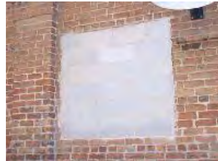
Damaged masonry should be replaced in kind rather than with another material.
