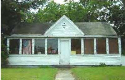
Inappropriately enclosed porch with glass and vinyl siding.
